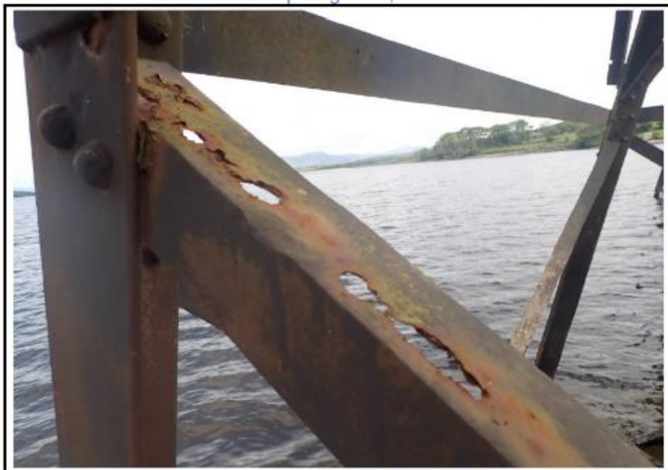
Photo 8: Section loss to bottom diagonal, trestle 3
